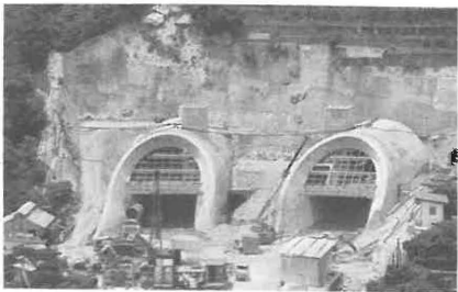
The Aberdeen tunnel is one of the major road projects expected to be completed next year. Page 18.
