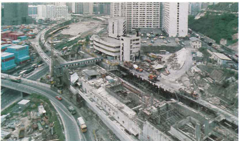
General view of the construction at Lai King Station, one of the five stations of the MTR's Tsuen Wan Extension.
